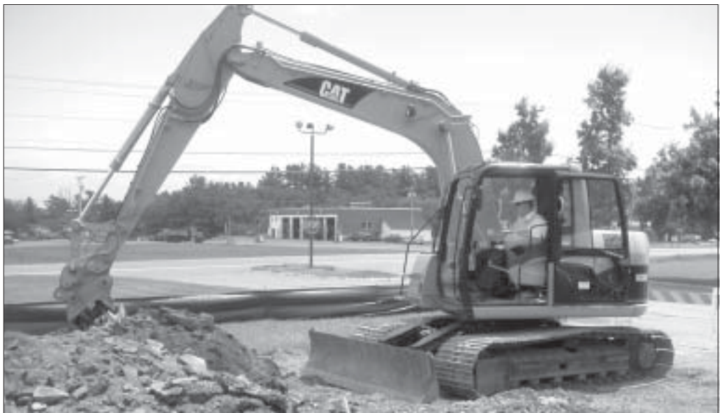
Daniel McPhee operates an excavator as students redo a portion of the UTC parking lot.
